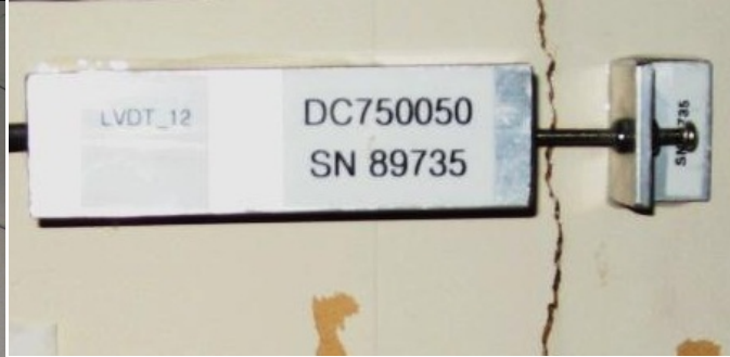
↑ a - Close-up of ceiling crack monitored by LVDT_12
