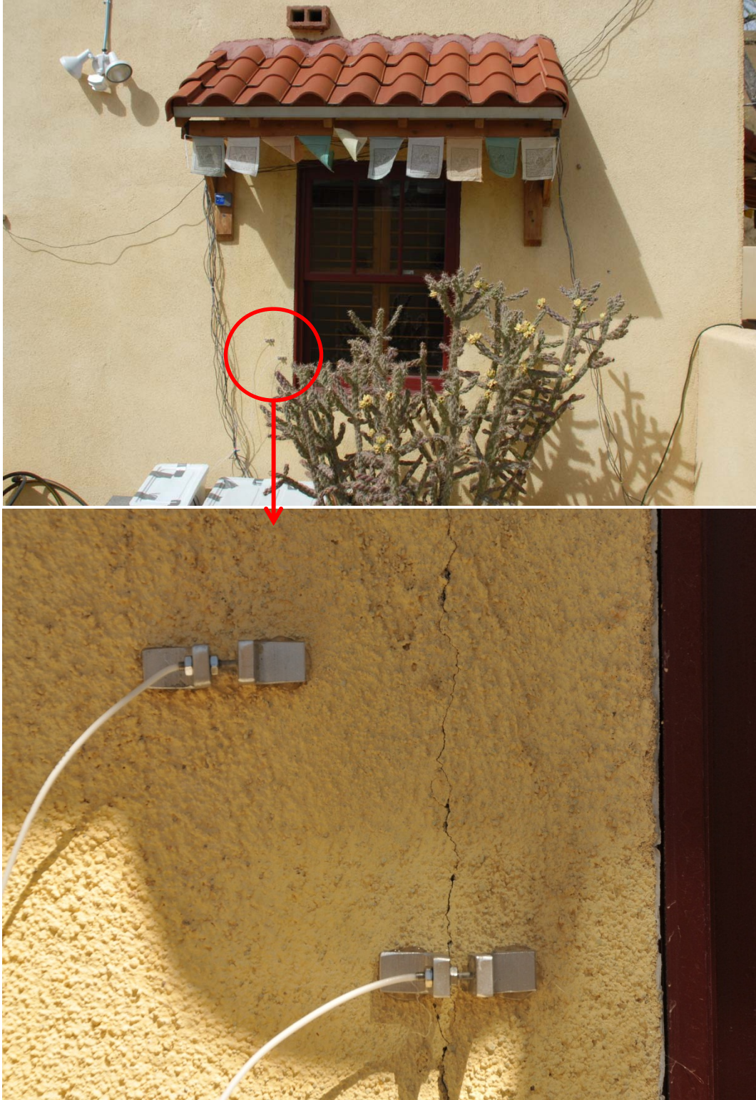
Figure III-5 - Crack displacement gauges mounted over an existing crack and un-cracked wall section
