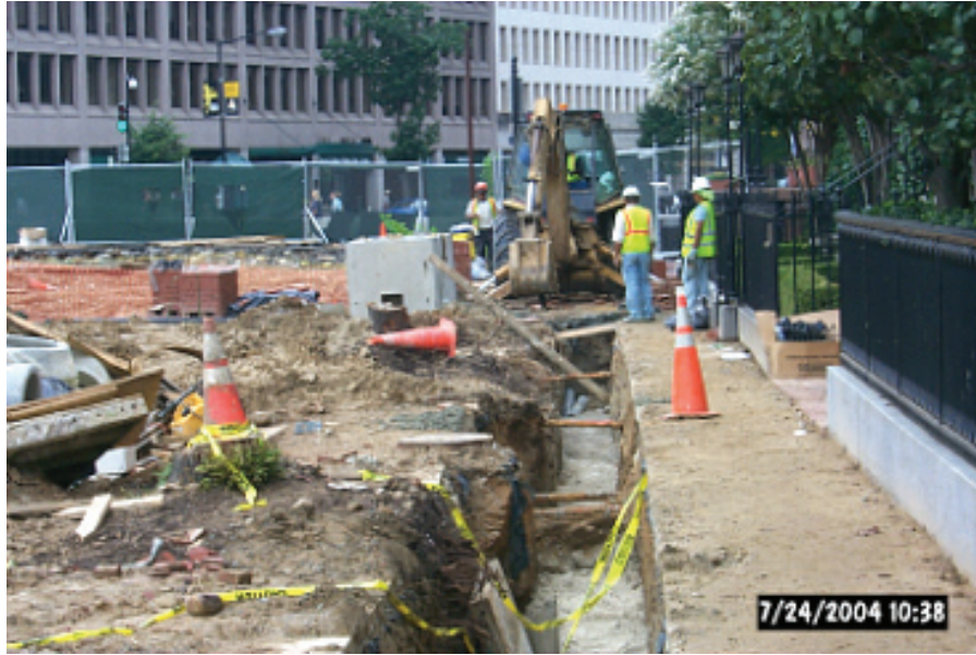
FIG. 1: Construction activities nearest Blair House showing trench excavation within several meters of Blair House. (Alvarez, 2004)
