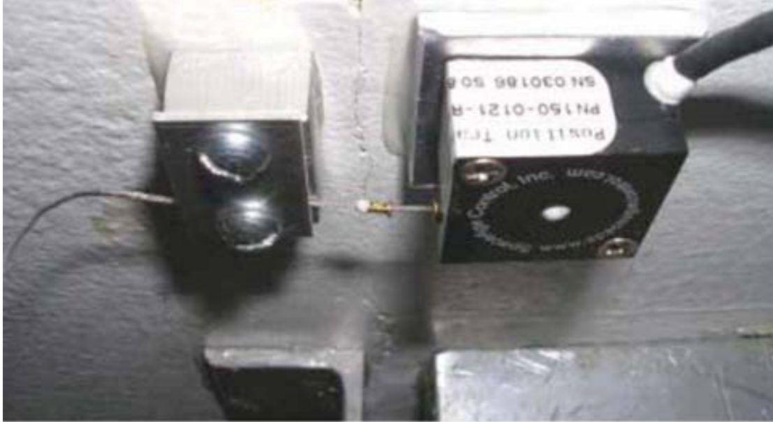
Figure E-8: Details of the potentiometric proximity sensor spanning the ceiling crack
