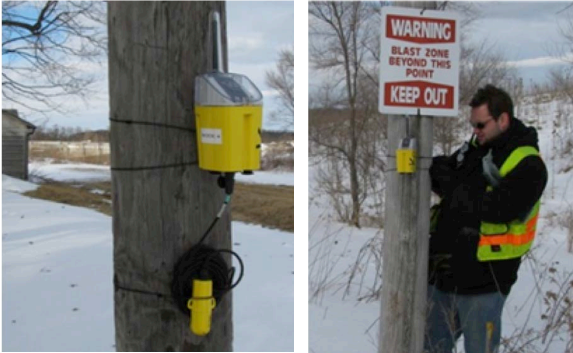
Figure E-3: Installation of exterior nodes. Left installation includes temperature and humidity sensor module below the node.
