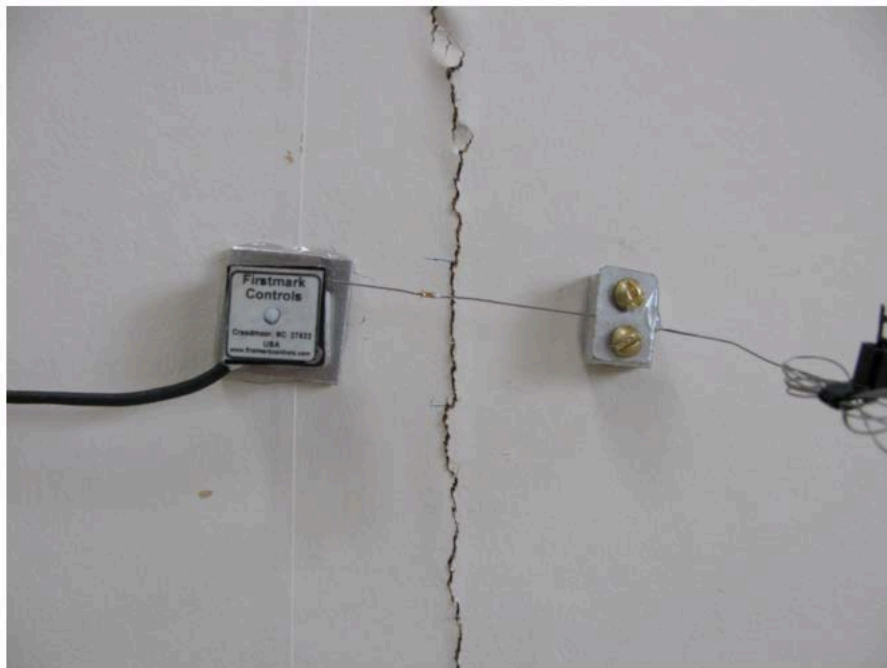
Figure D-14. Close-up of string potentiometer across ceiling crack.
