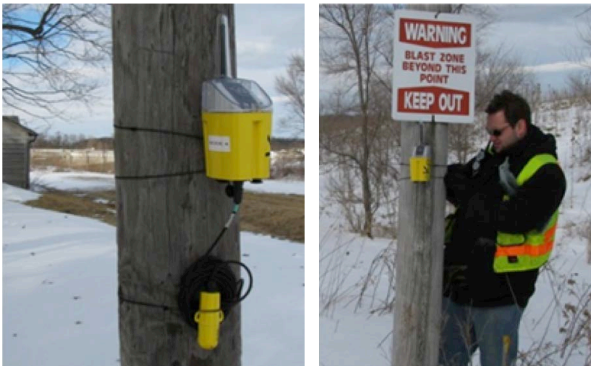
Figure D-15. Installation of exterior nodes. Left installation includes temperature and humidity sensor module below the node.
