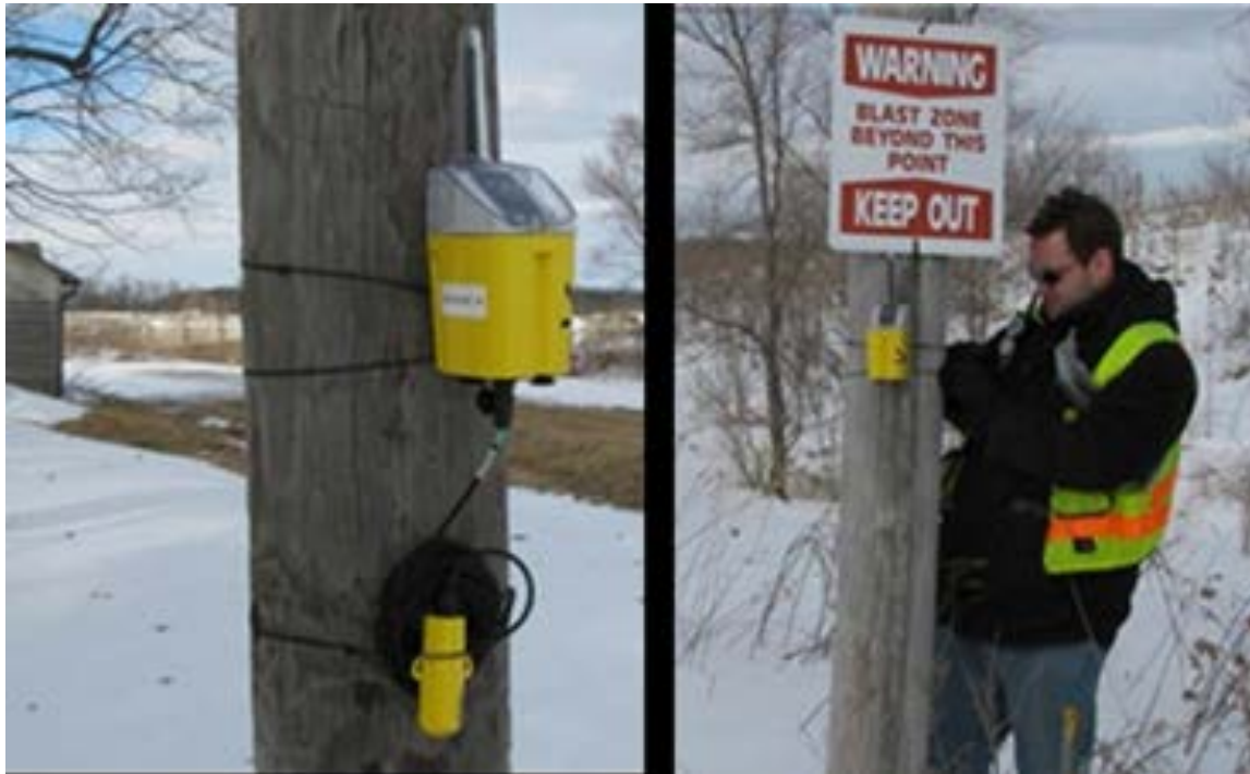
Figure DS-1: Installation of the weatherized motes for transmission of data from the test house to the structure with the internet connection. Yellow device below the mote on left is a temperature probe that accesses the mote from a port that also allows attachment of the crack response gauge, which illustrates the flexibility of these newer designs.
