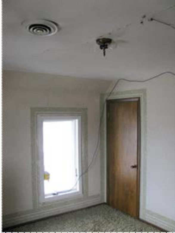
Figure E-6: Context of node 3 and ceiling crack sensor. A close-up photograph of the ceiling crack and potentiometric proximity sensor is shown in Figure E-8.
