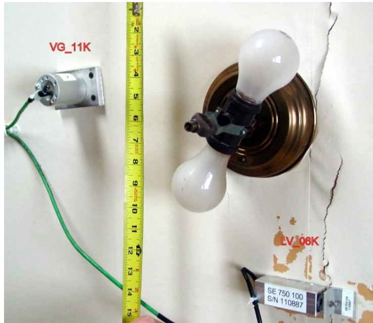
Figure 24: Bedroom Ceiling Sensors
