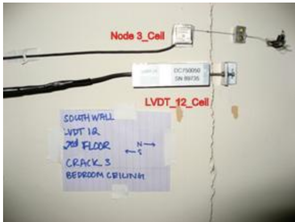
Figure 4: Ceiling Crack Bedroom with Sensors
