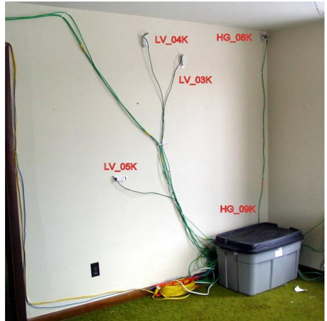
Figure 23: Interior E-W Wall Sensors
