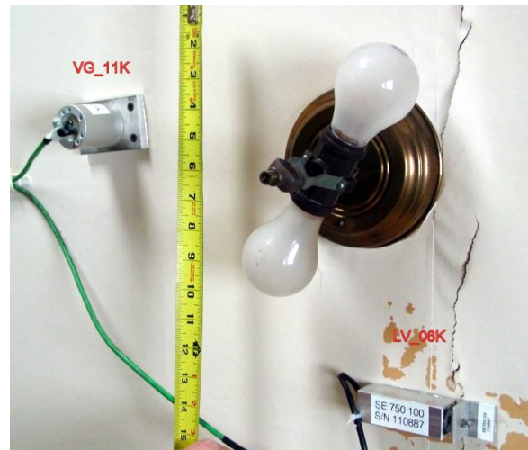
Figure 5: Ceiling Crack Bedroom with KEP sensors
