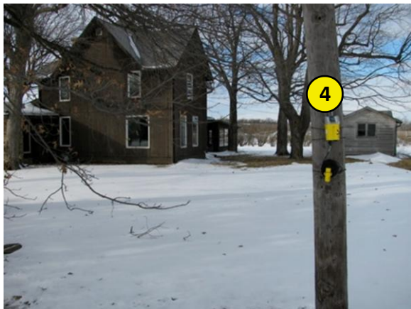
Figure 2.4 - Node 4 as relay point on telephone pole
