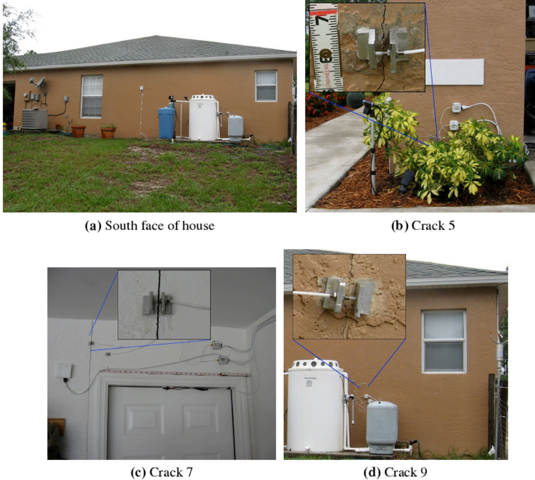
Figure 5: General locations of crack displacement transducers, with insets showing detail of cracks and sensors
