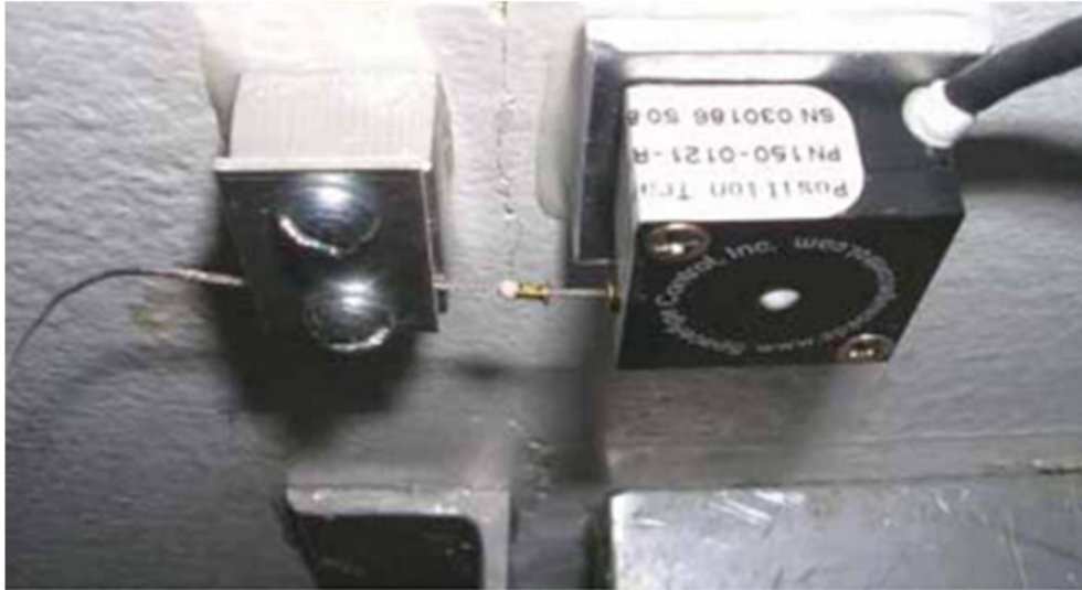
175 176 Figure 8: Details of the potentiometric proximity sensor spanning the ceiling crack
