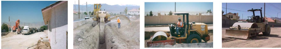
Figure 1 (L-R) Test House w/ Hitachi trackhoe, Tesmec chain trencher, Dynapac small and Ingersoll Rand large vibrating rollers.
