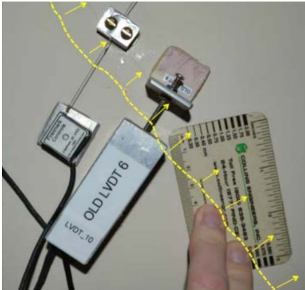
Figure 3: Null gauge with arrows pointing to the visible crack and an offset dotted line indicating the crack contour. The crack gauge shows an approximate crack width of 0.20 mm.
