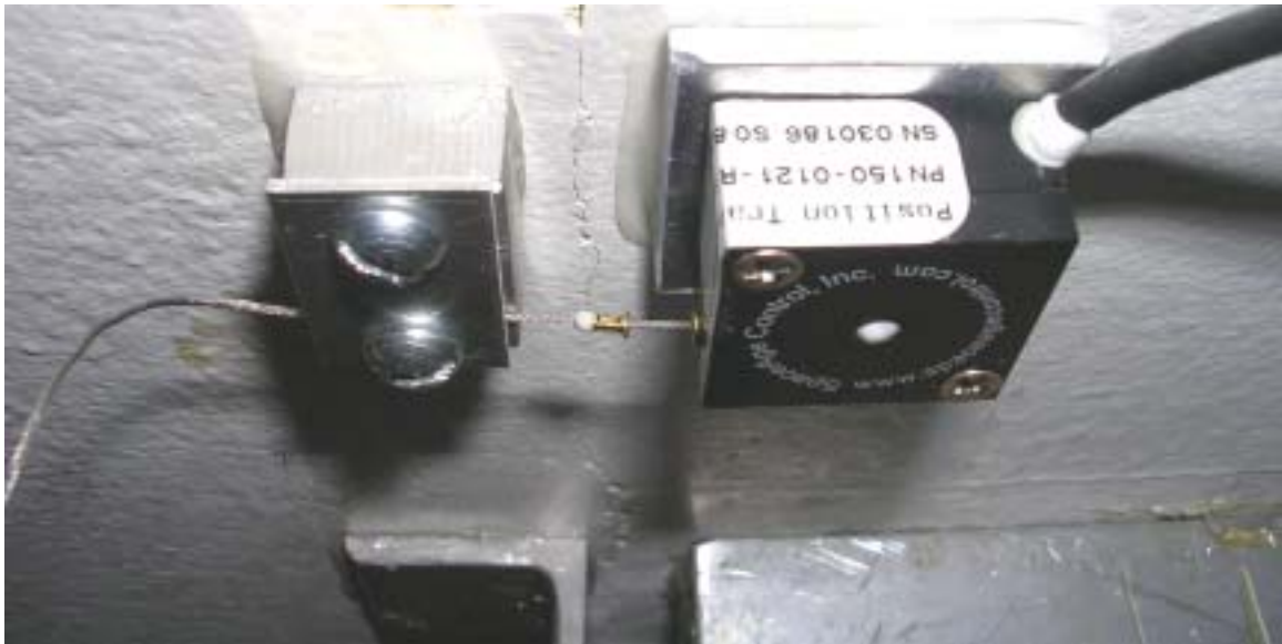
Figure 3.6: Potentiometer and LVDT glued on the ceiling crack of the test house in Milwaukee
