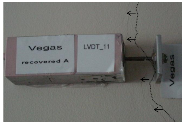
Figure 3. Overall views of the wall-mounted crack sensors
