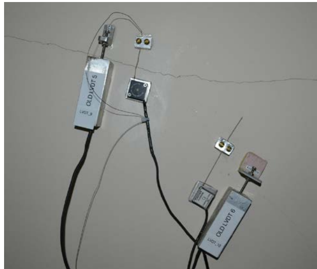
Figure 3. Details of the shear crack and crack gauges (LVDT and potentiometer) and null gauge before appearance of the crack.
