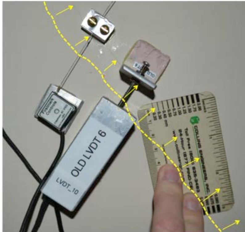
Figure 7: Null gauge with arrows pointing to the visible crack and an offset dotted line indicating the crack contour. The crack gauge shows an approximate crack width of 0.20 mm.
