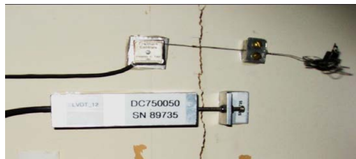
Figure 4. Details of the ceiling crack and crack gauges (LVDT and potentiometer).
