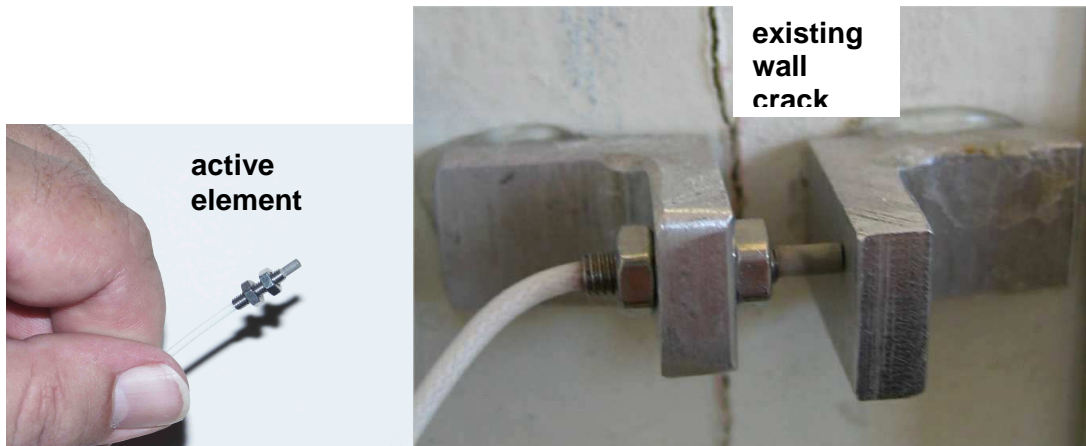
Figure 5 Displacement gage system used to measure opening and closing of an existing wall crack (above) and close-up of mounted crack gage (below)
