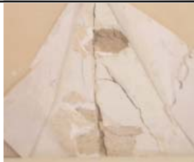
interior plaster and lath crack 3
