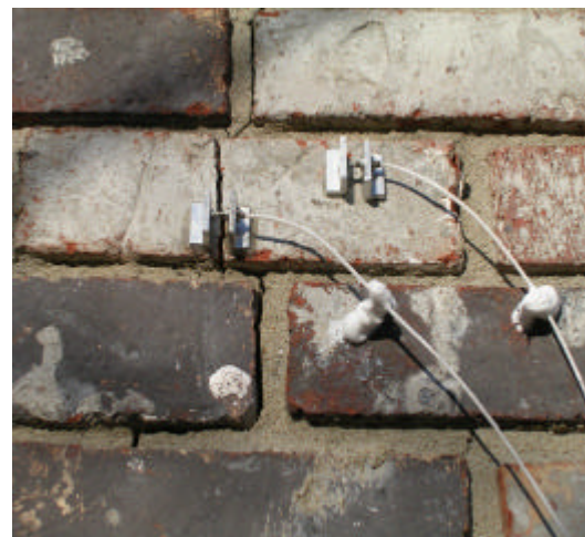
Figure 2.5 Photographs showing the location and detail of each of the three monitored cracks
