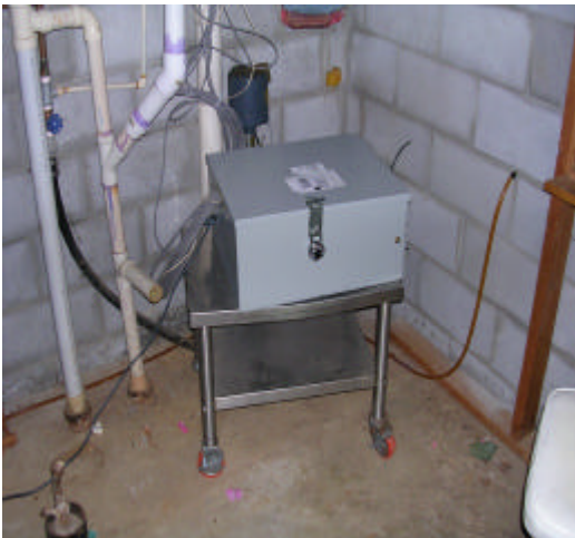
a) Data monitoring secure enclosure houses eDAQ in corner of basement
