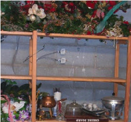
b) Indoor Basement Crack
