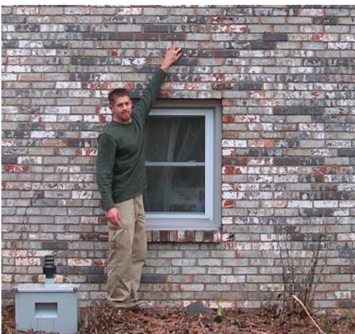
c) Exterior Crack
