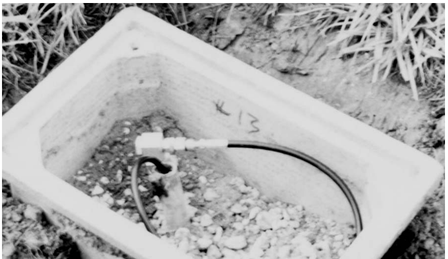
Figure 10. Protective enclosure for connection between a sensor and a connecting cable
