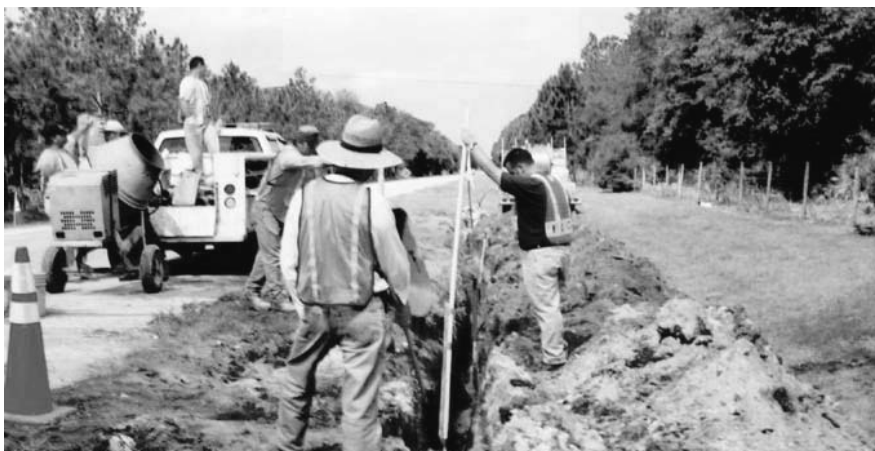
Figure 1. Installation of horizontal TDR sensor cable in a grouted trench over a stabilized sinkhole
