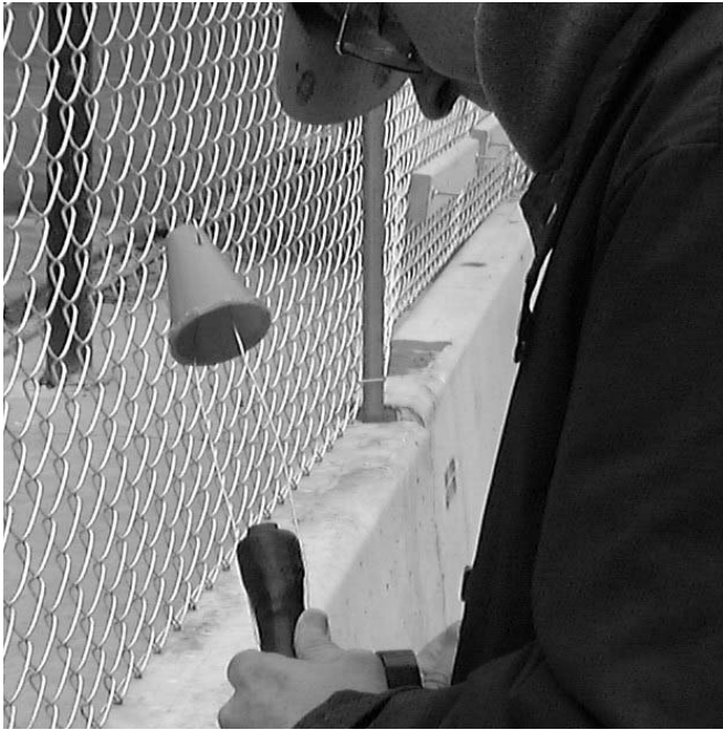
Figure 8. View of the sealed end tip of a flexible TDR sensor cable also fitted with a plastic cone to catch the PVC grout tube for insertion
